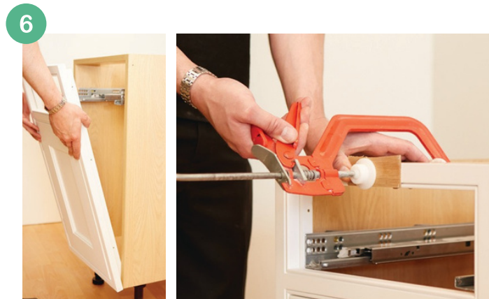
6 Once the adhesive has dried, position the frame against the carcass. The bars should rest on the bottom shelf for ease of installation. Protect the frame and use a clamp to hold against the carcass.
